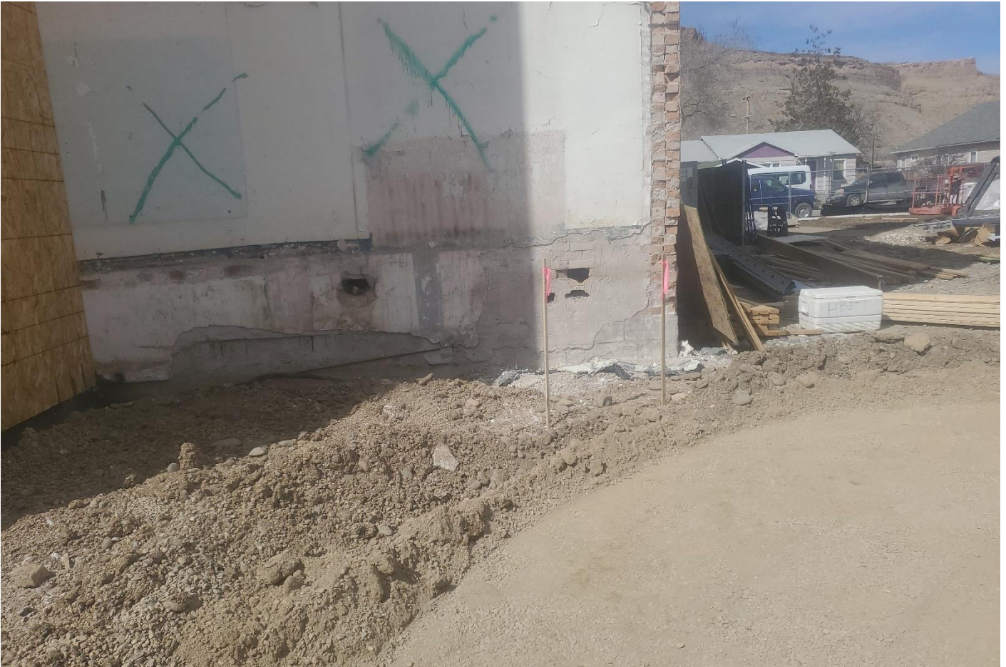
Exterior wall with additional unstable brick needing additional stabilization.
